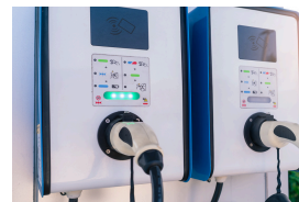
EV Charging, OBC, EVSEs
