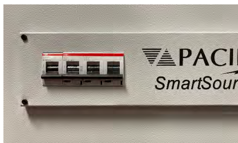
Figure 5-3: Mains CB in OFF (lower) Position
