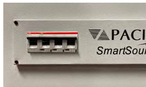
Figure 5-4: Mains CB in ON (upper) Position
