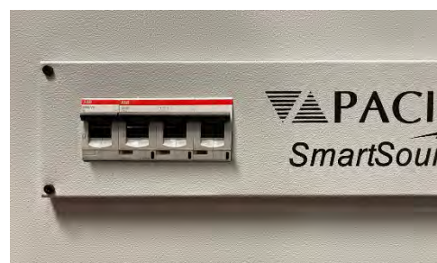
Figure 5-4: Mains CB in ON (upper) Position
