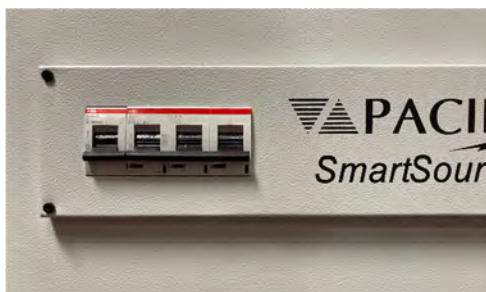
Figure 5-3: Mains CB in OFF (lower) Position
