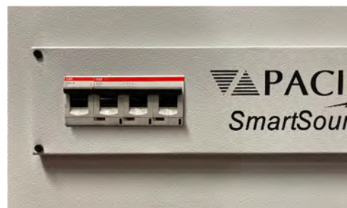
Figure 5-4: Mains CB in ON (upper) Position
