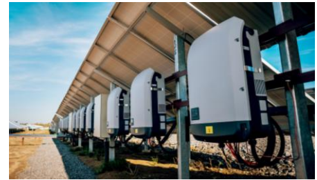
Solar PV Inverters
